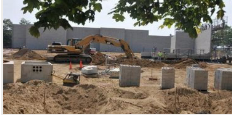
Work continues on a Circuit City store due to open in Hyannis in the coming months. It is one of 45 to 55 stores the company will open this year. Cape Cod Times/Steve Heaslip
